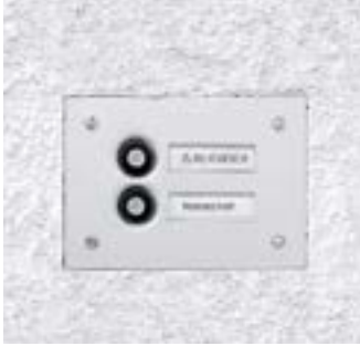
Sole condition: A bell system, in this example for a two-family home
